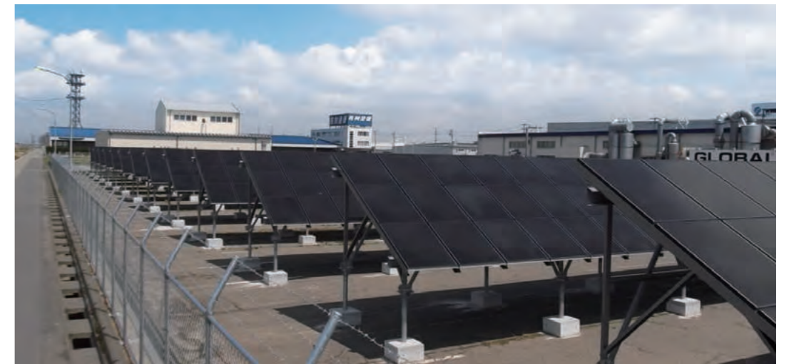
Utilizing renewable energy in its business operations, Twinbird installed solar power generation systems on the premises of its Head Office, with their maximum output totaling 250kW.
